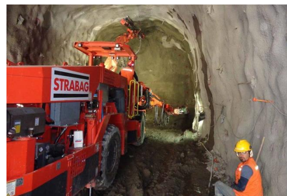
Alto Maipo power plant
