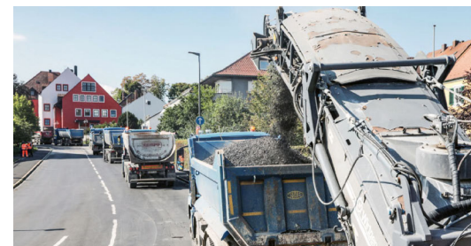
Around 3,180 t of asphalt were installed over a length of 975 m using a total of thirty semitrailers.
